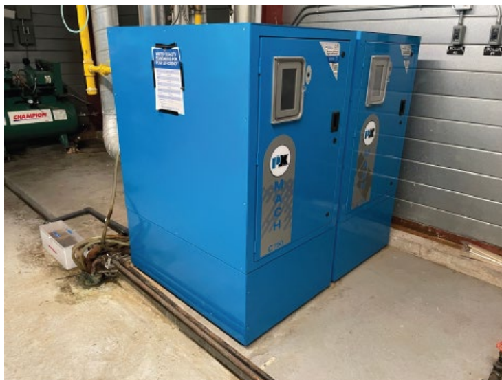
15 Figure 2: Photos of HVAC
