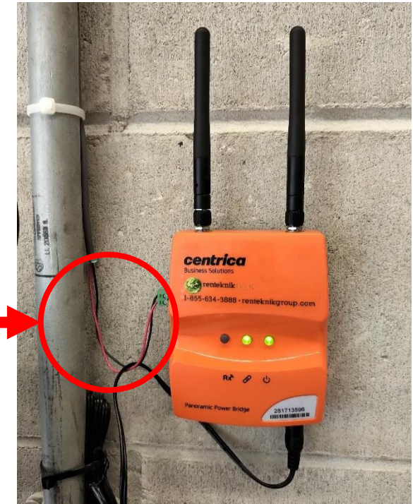
Communication Bridge – Pulse Input
